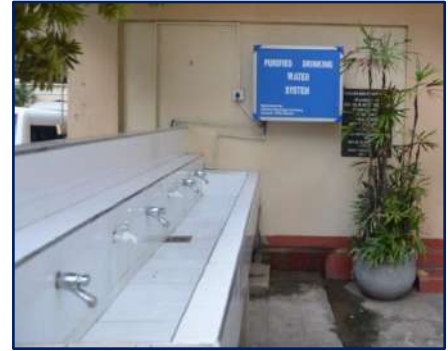
Purified Water System
